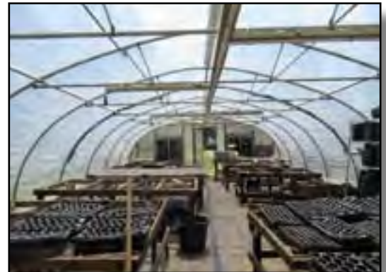
Greenhouse after irrigation installed; fans, heaters and sunscreen up and running.
